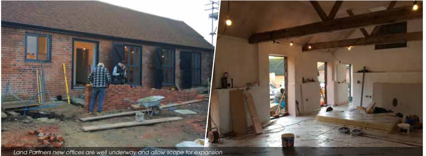
Land Partners new offices are well underway and allow scope for expansion
